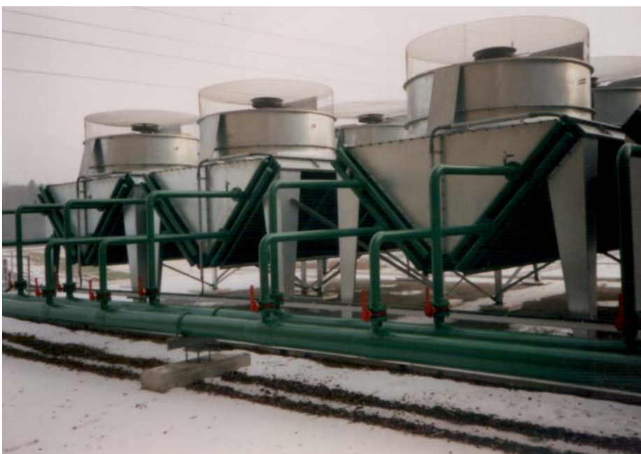
Double block cooling devices ECODYNE AG with six impeller ventilators for ABB gas turbine in power plant
