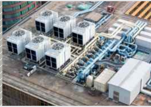
Vibration protection for air-conditioning system
