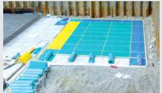
Building foundation bearings
